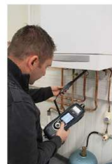
Ambient CO checking
